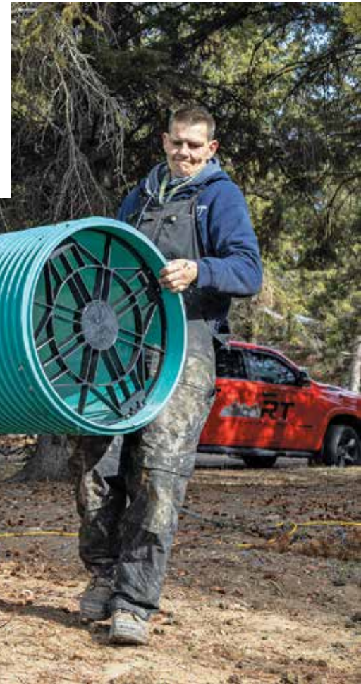
▼ RT Septic employee Trevor Walker carries tank riser material during an installation project. (Photo by Stephen Defoe)
