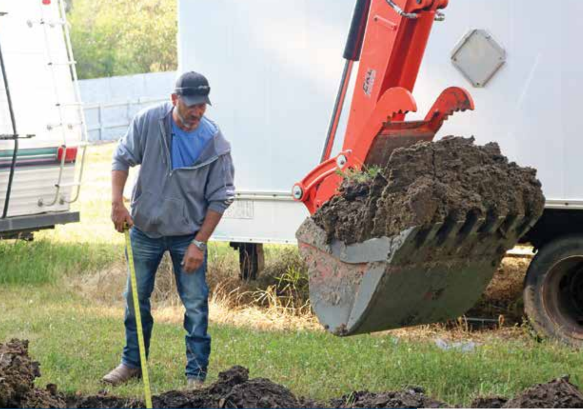
◀ Tipple checks the depth of an excavation before getting back on the excavator to finish the job. (Photo courtesy of Kubota Canada Ltd.)
