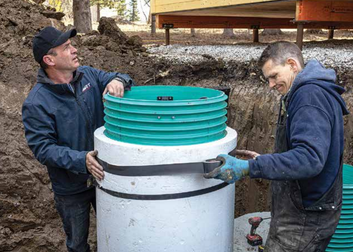
◀ RT Septic owner Rick Tipple and employee Trevor Walker work on installing AWS Riser Wrap Insulation around a green ultra-rib pipe. (Photo by Stephen Defoe)
