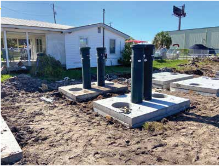
◀◀ The Anua PuraACE reactor pods getting prepped before installation in the aeration tanks.
