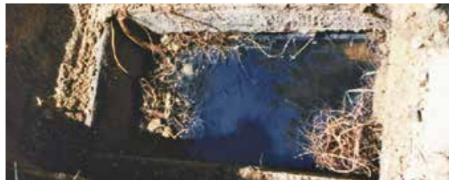
▼ Tree roots are clogging a distribution box.
