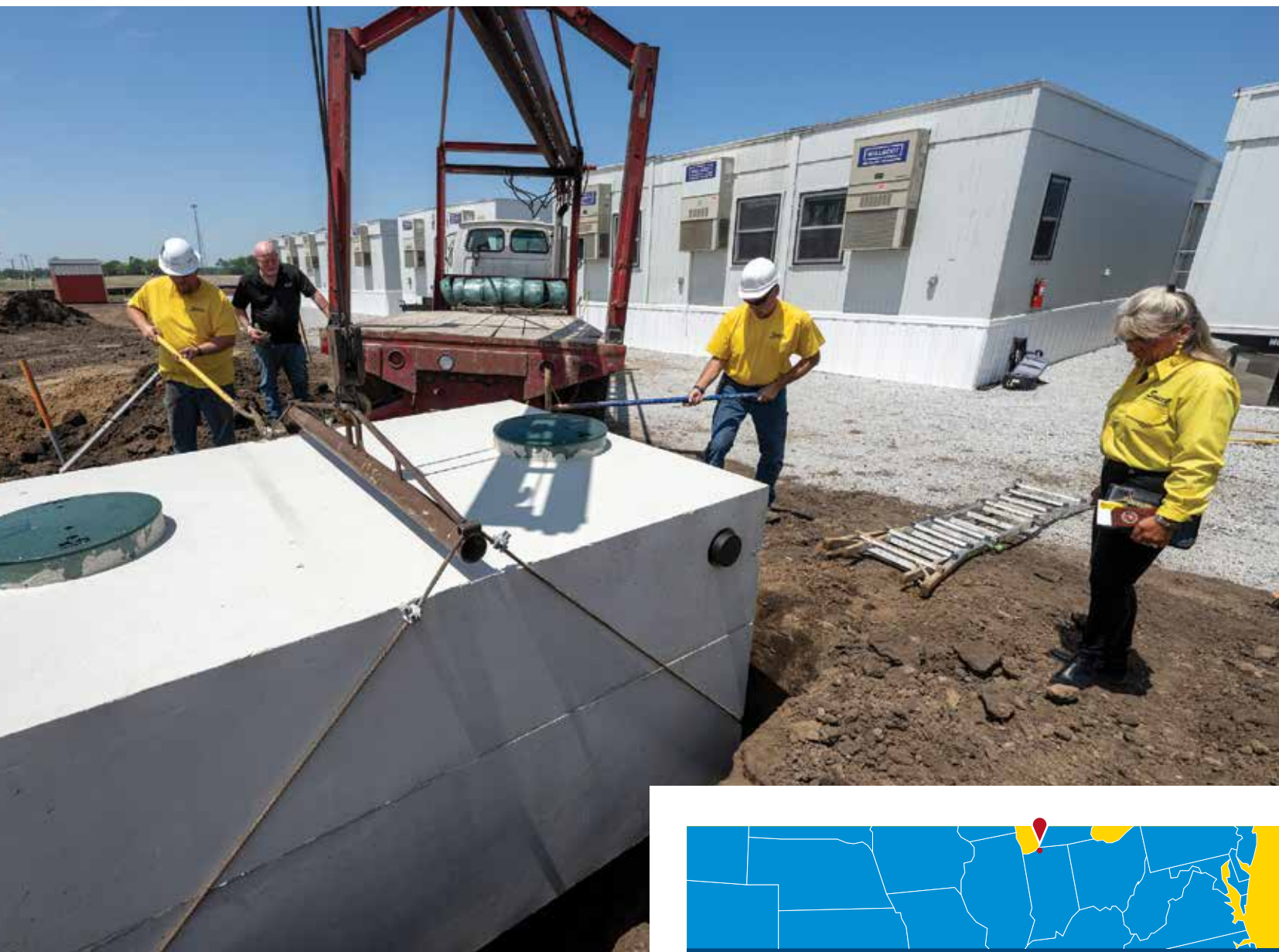
▲ Left to right, Cody Houseknecht, a delivery driver and Jon (right) Houseknecht maneuver a septic tank into place during a recent install project. Gale Houseknecht, far right, observes. (Photos by Mark Lebryk)
