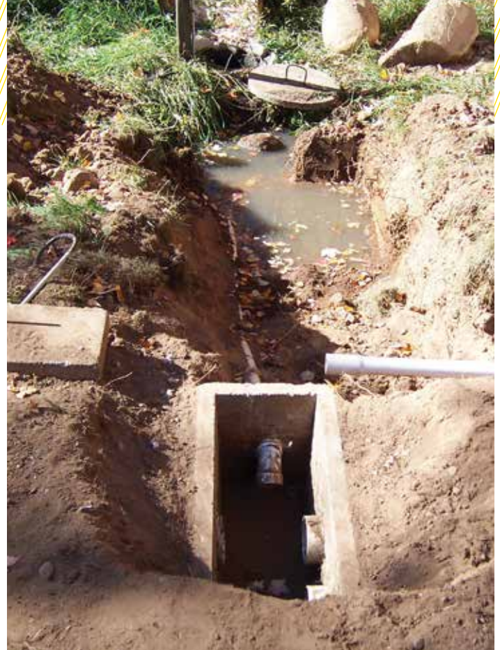
▲ Mid-repair, the existing pump tank and pump line into a distribution box are being replaced. (Photos courtesy of Sara Hager)
