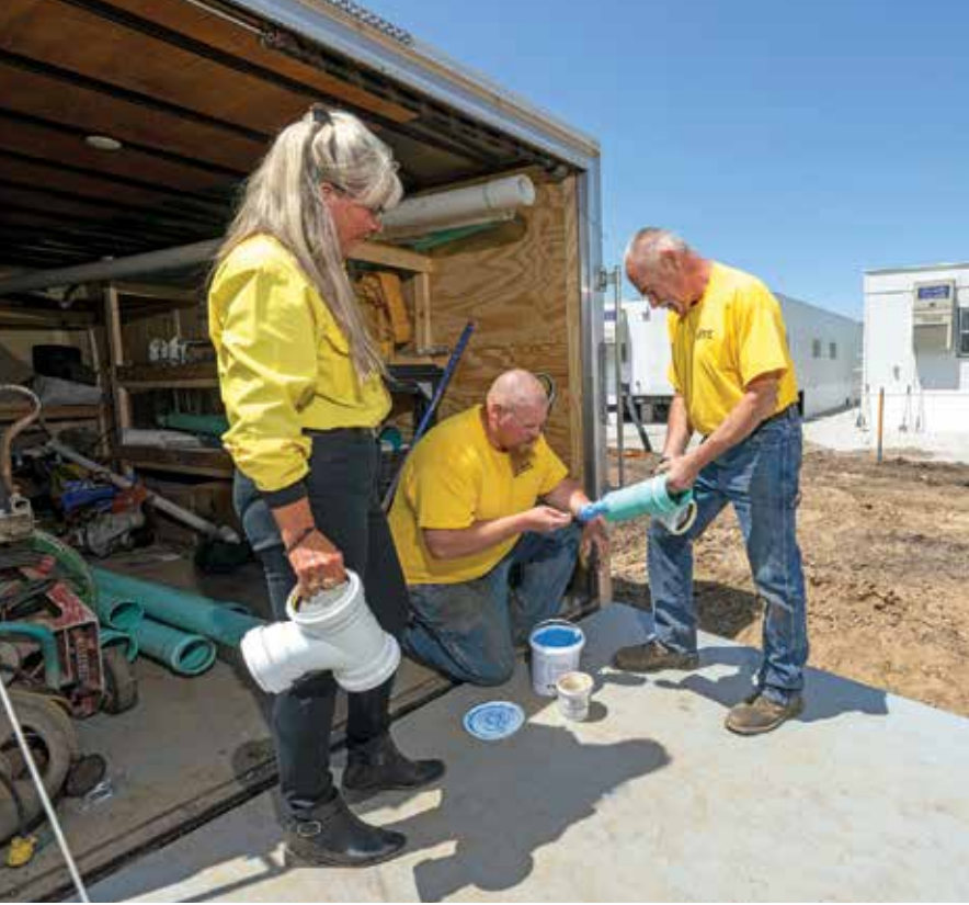
◀◀ On location at an install project, the Houseknechts assemble parts needed for a pipe run.
