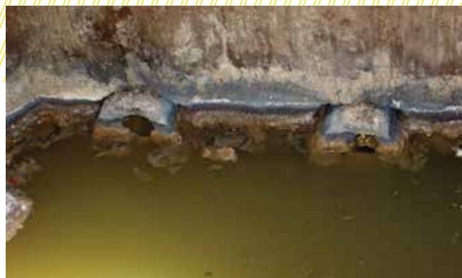
▲ The view inside a dirty distribution box.
