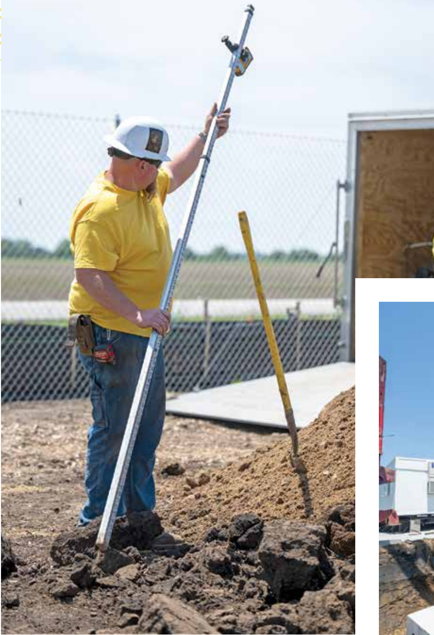
▲ Cody Houseknecht takes down a grade rod used to level a septic tank.
