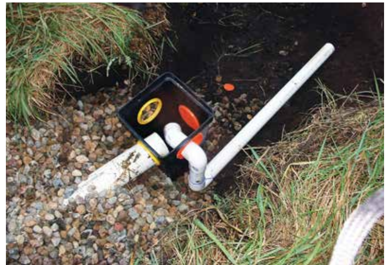
▲ A gravity distribution box is being installed. (Photo courtesy of Sara Heger)
