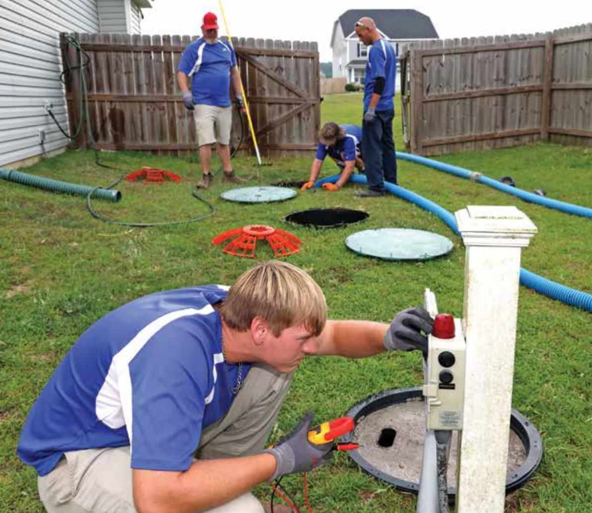
◀ Hunter Creech checks the voltage at a SJE Rhombus NEX Series pump control panel as Stacy Creech and crew service and clean a home septic system.
