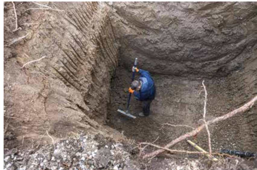
▲ This unidentified worker is at the bottom of an estimated 15-foot-deep septic tank excavation with no shoring, a clear OSHA violation. This photo was submitted to Onsite Installer . We wouldn't normally run it in the magazine, but do so here to stress the importance of following safety rules. We alerted the installer contractor about the violation on the job site.
