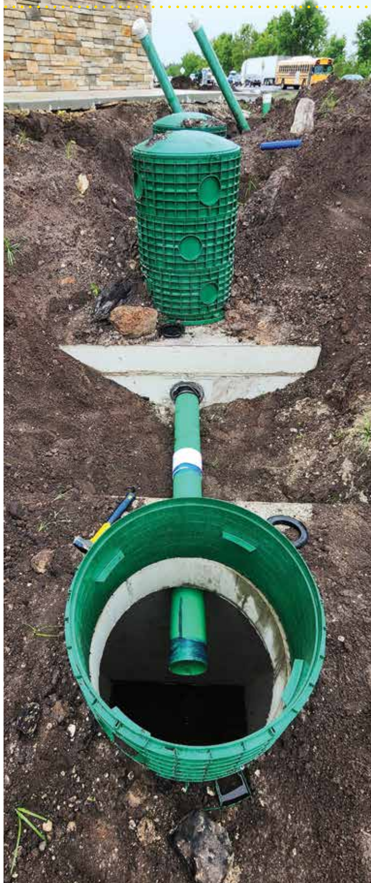
▲ Two 1,050-gallon H-20 traffic-rated concrete grease interceptor tanks set in series with TUF-TITE risers and lids. (Photos Courtesy of Greg Mayfield)
