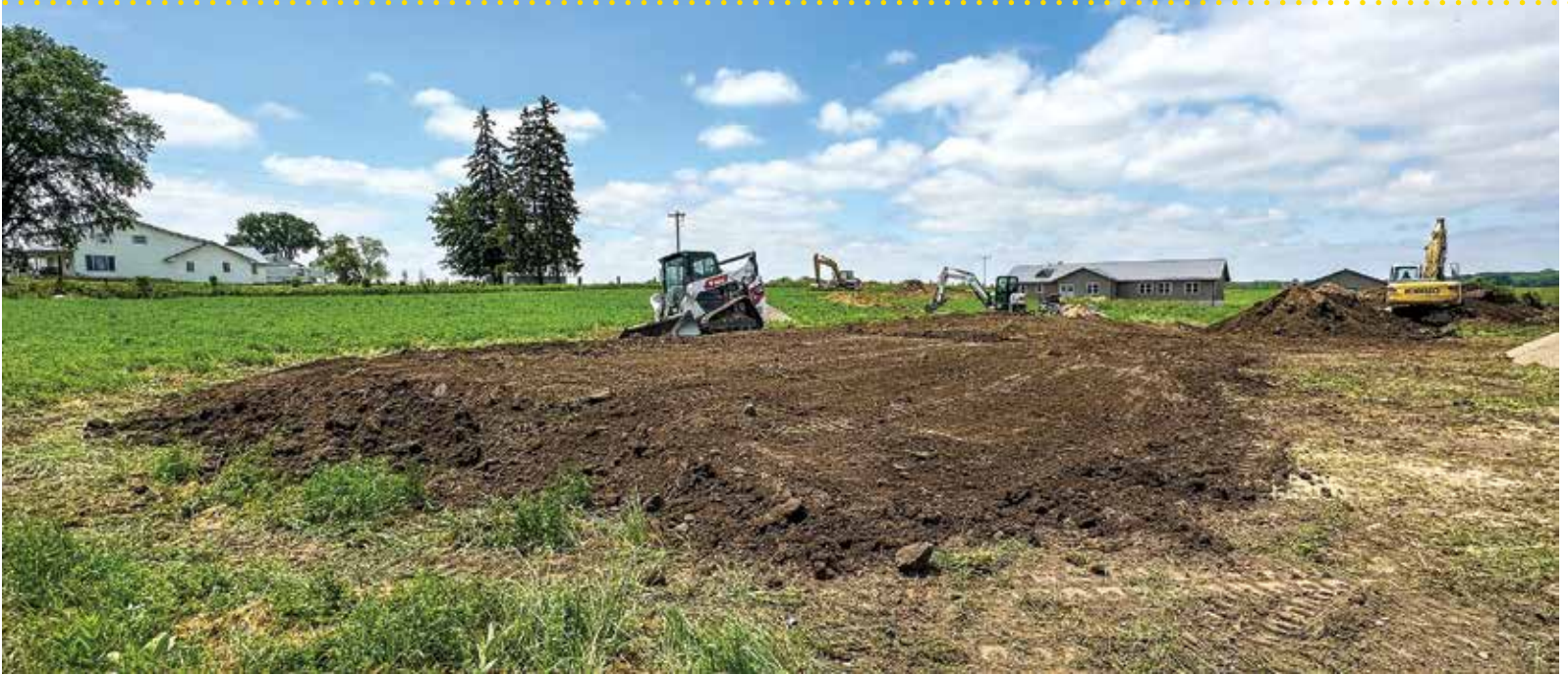
▲ Anthony Bontrager in the Bobcat E55 compact crawler excavator throws topsoil on the Presby treatment bed, while Jay Bontrager uses the Bobcat T76 compact track loader to level it.
