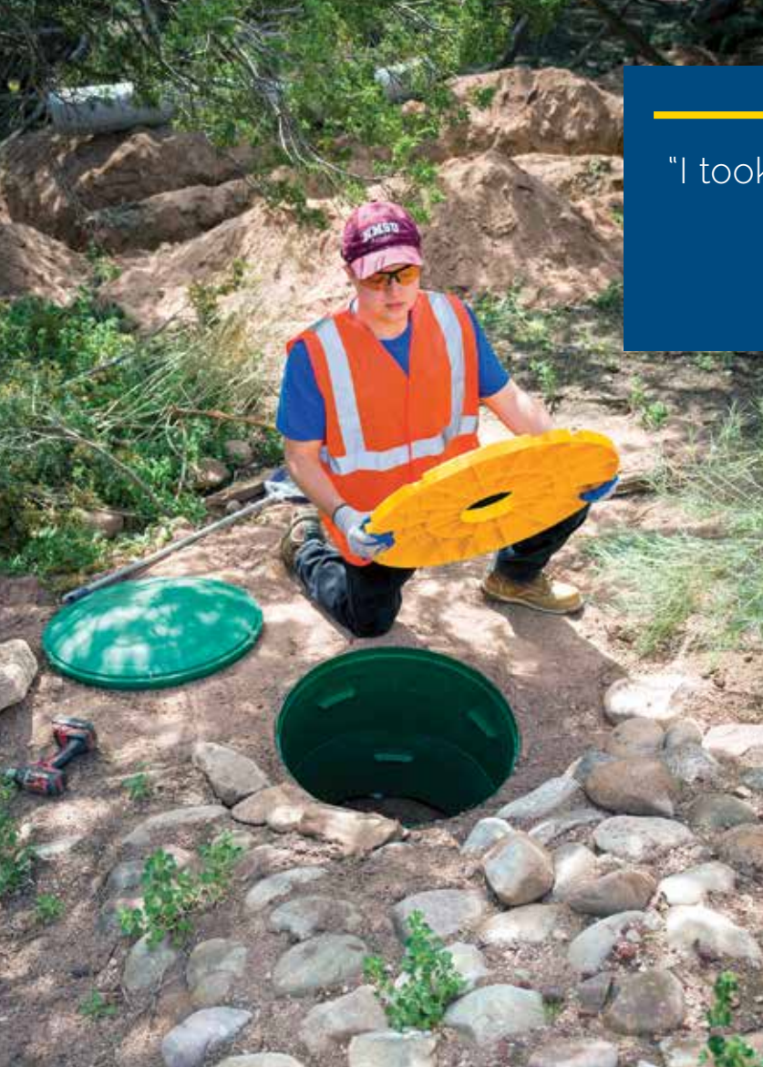
▲ Gino Dotson adds a Safety Lid from TUF-TITE to a new septic system. The yellow inner lid offers added protection to prevent people from falling into the tank.
