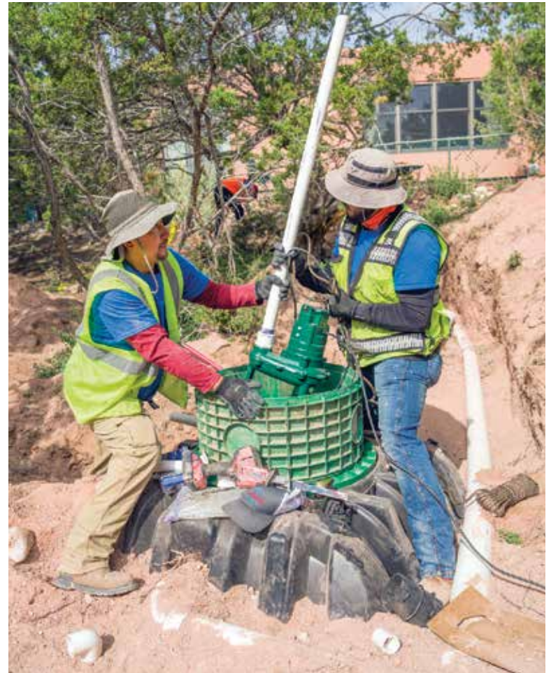
▲ From left, Giovanni De La Paz and Juan Alvidrez lower a Zoeller pump through a TUF-TITE riser and into an Infiltrator Water Technologies tank during a system installation.
