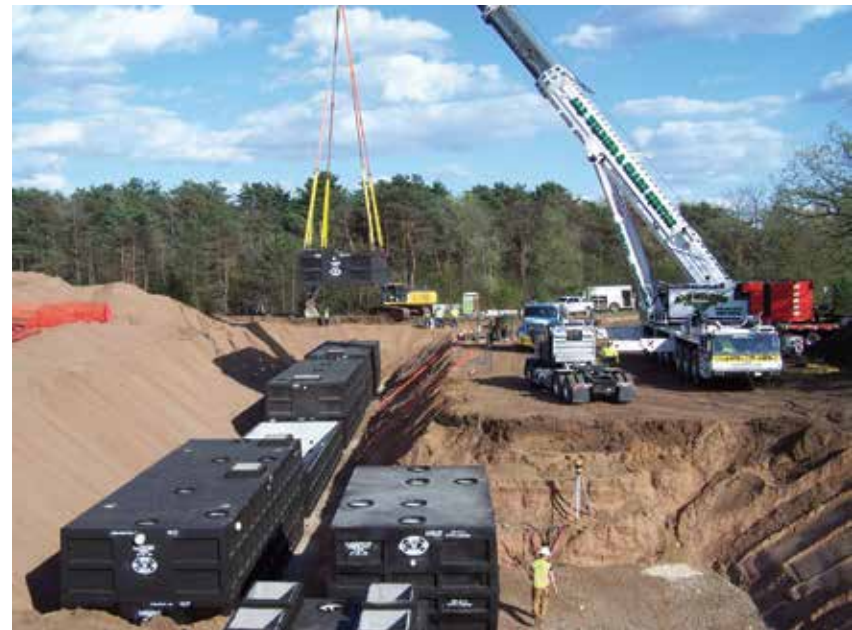
▲ Workers install a series of septic tanks to handle a peak daily flow of 55,000 gallons at the front end of a cluster system in Sara Heger's community of Afton, Minnesota. (Photos by Sara Heger)
