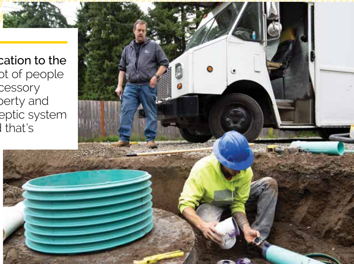
▲ Tom Purdum oversees an OSCAR septic installation he designed in Edgewood, Washington. The installer is Lewis Gregg of A-Bell Excavating of Puyallup, Washington.
