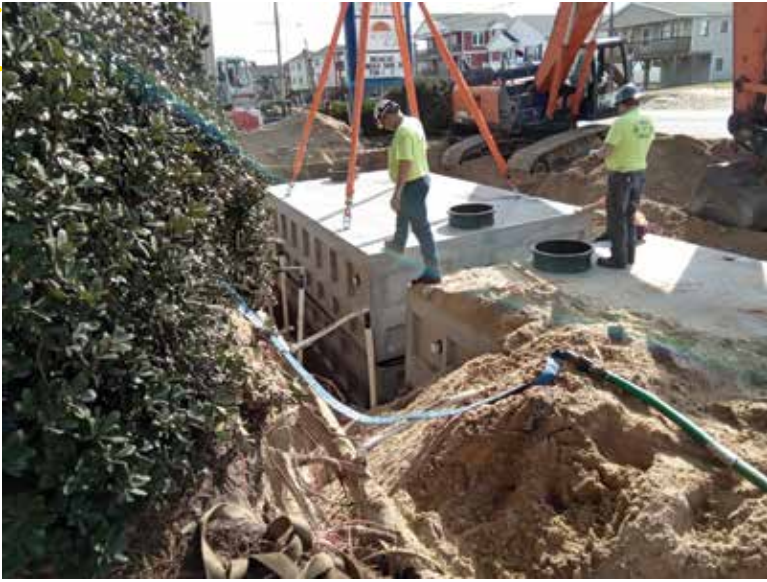
◀◀ Jon Harris and Wieser Concrete field crews make sure the tank halves are lined up and in the proper position.
