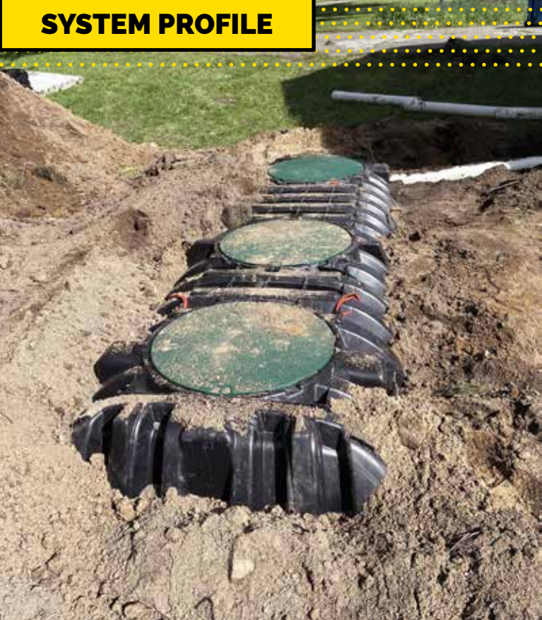
▲ Proper backfilling of a tank is one of the lessons taught at field days of the Indiana Onsite Wastewater Professionals Association. Here the Infiltrator IM-1530 poly tank sits in its hole at Pam's Promise in Crawfordsville, Indiana.
