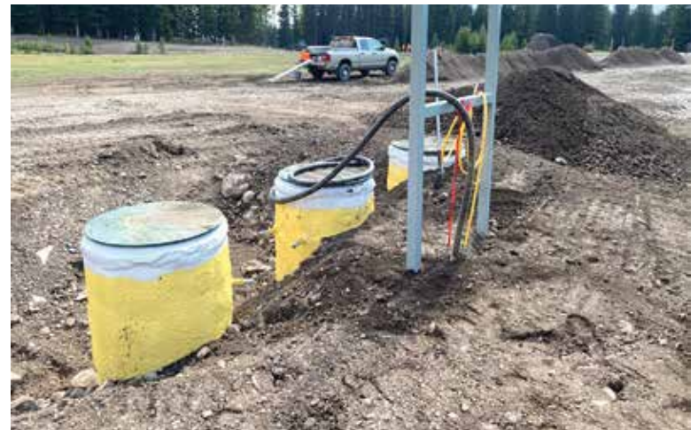
Yellow insulation has been sprayed over the exterior of these risers before backfill to prevent freezing. (Photo courtesy of Clayton Foster)
