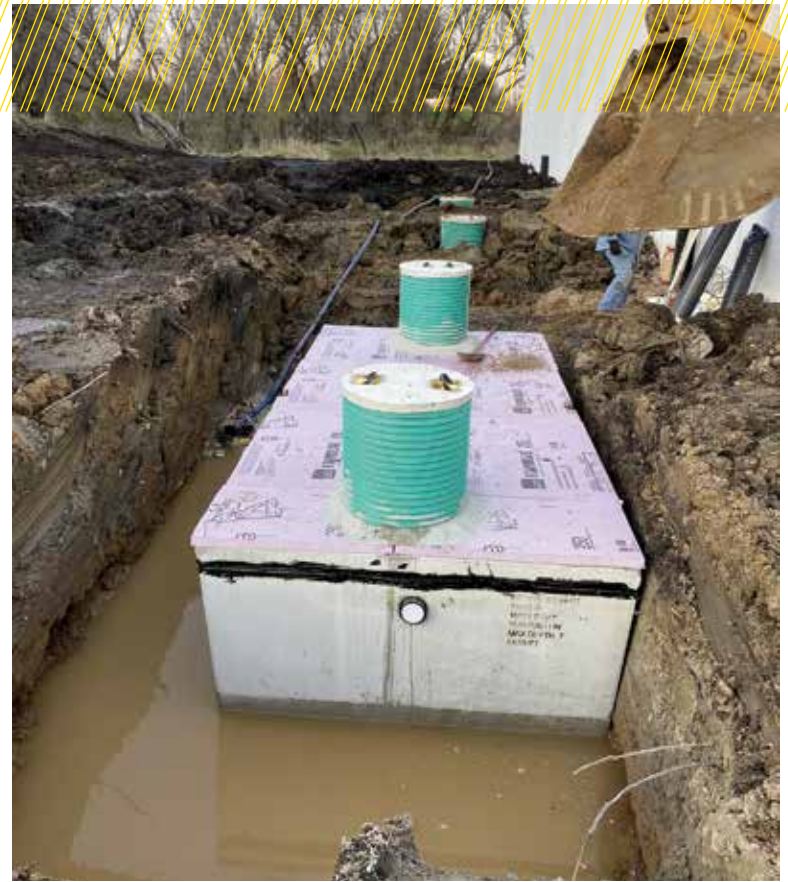
▲ Pink foam insulation is enough to prevent freezing in this tank that will be buried in a shallow excavation. (Photo courtesy of Tim Haeg)
