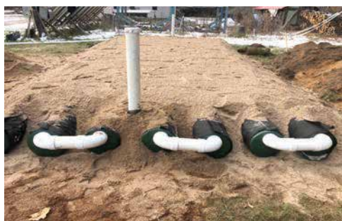
First AES installation in Wisconsin, November 2019
