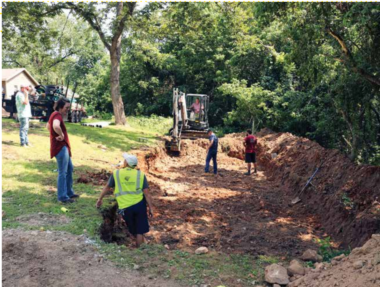
◀◀ The crew from BBB Septic and Portable Toilets, of Bentonville, Arkansas, builds the sloped sand bed for the day care center. Brook Cannedy runs the mini-excavator, while Kevin Phipps, right, waits to check depth, and Isaiah Muldoon, second from right, watches the progress. Kyle Krievans of the Arkansas Department of Health, left, observes while Erica Long, second from left and also from the state health department, talks to Curtis Cluckey of Infiltrator Water Technologies, third from left.
