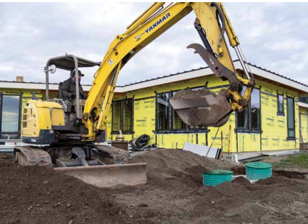
▲ At the site of a new system installation, Ben Miller uses a Yanmar excavator to backfill a new concrete septic tank.
