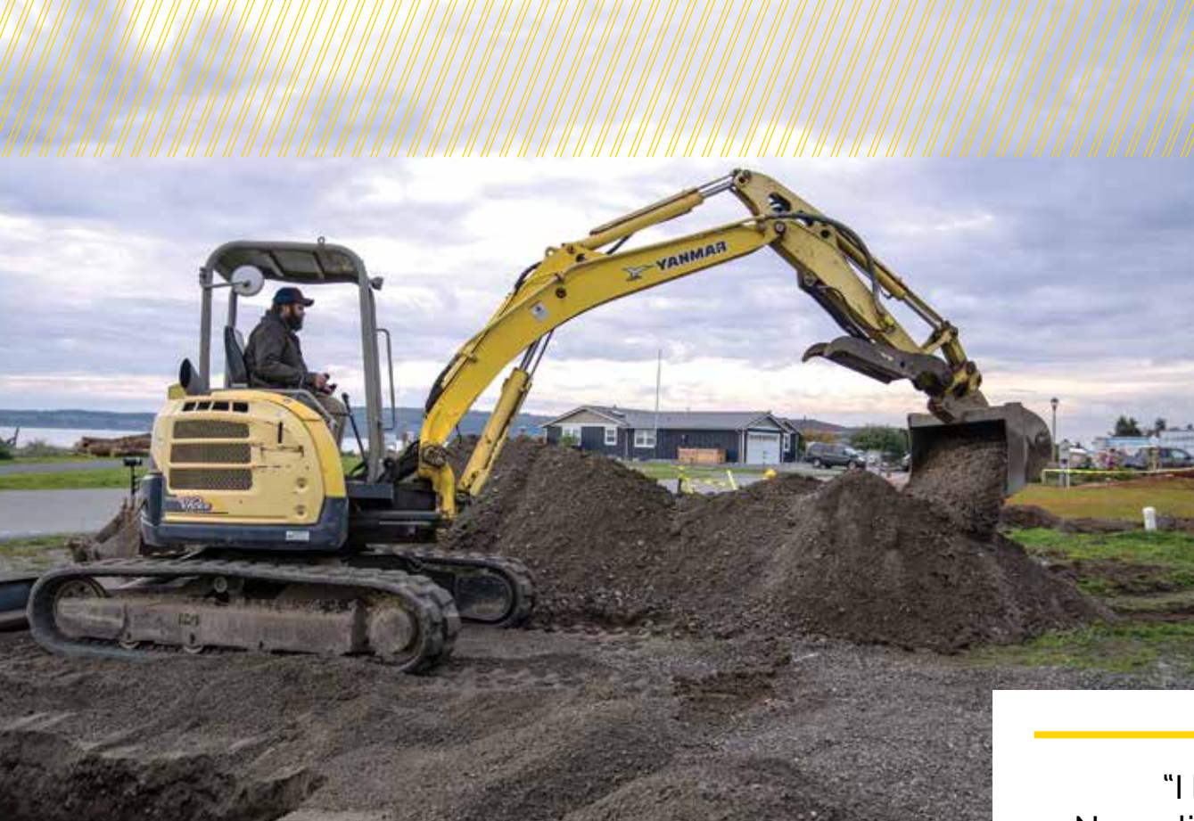
◀◀ Ben Miller excavates a hole for a new septic tank on a residential job in Oak Harbor, Washington.
