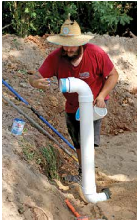
◀◀ Isaiah Muldoon, of BBB Septic and Portable Toilets, sets up the vent pipe that will move air through the Infiltrator AES pipes.
