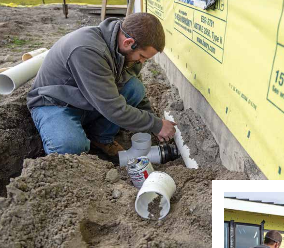
◀◀ Seth Miller tightens a fitting on a clean-out being installed ahead of a line from the house to the septic tank for a new-construction system.
