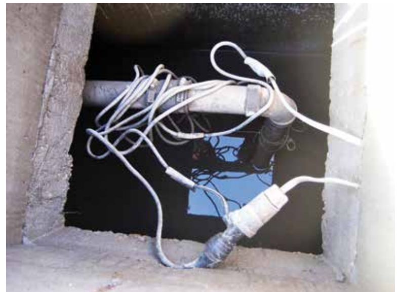
⚠️ Improper electrical connections inside a pump tank. (Nicholas Dykes photo)
