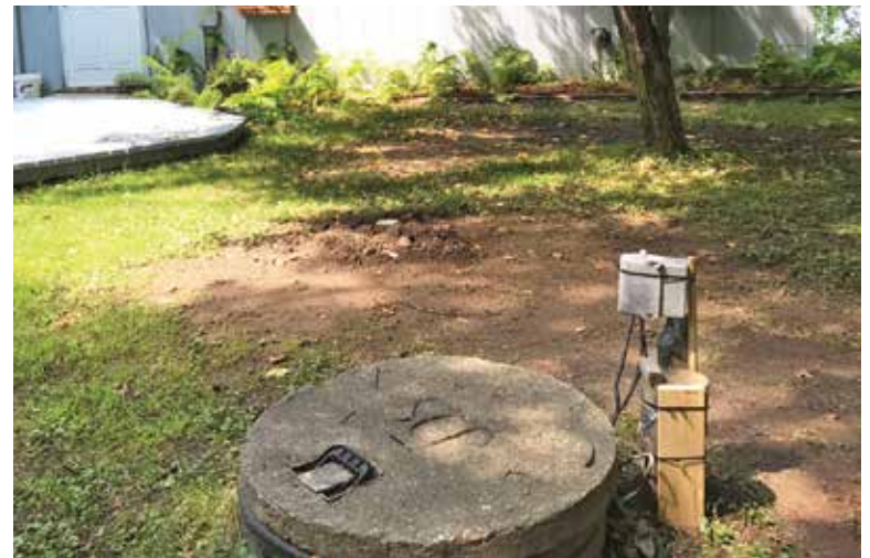
⚠️ This is an example of an inadequate installation of pump controls. (Sara Heger photo)
