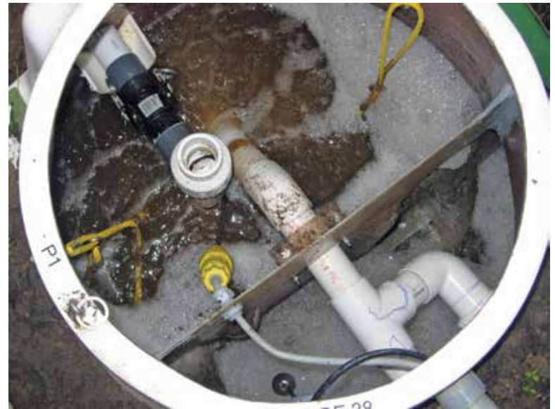
▲ A Cromaflow sequencing batch reactor from Cromaglass Corp. using submersible pumps to provide air and mixing with a venturi system receiving air through intake pipes from the atmosphere. (Photos courtesy of Sara Heger)
