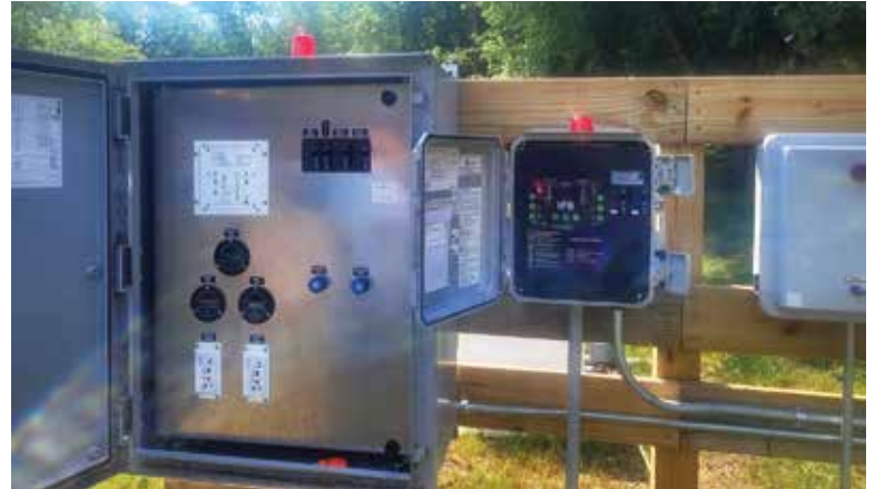
▲ Another installed SJE Rhombus system. These time-dose panels are for a septic system at a summer camp including a dining hall.
