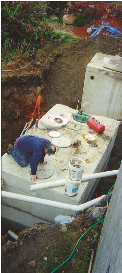
Jim Stevens of E.F. Shea Concrete Products prepares to vacuum-test the septic tank.
