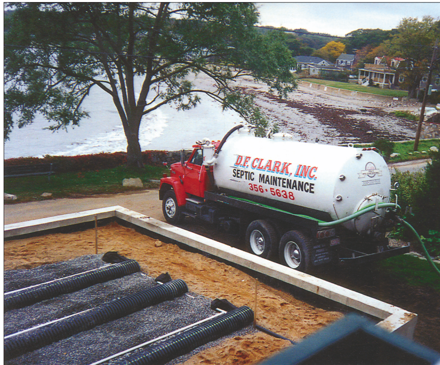
A septic hauler pumps out the original cesspool for the property in Gloucester, Mass. The cesspool was located on the neighbor's property. Photographs by Marcia Noga.
