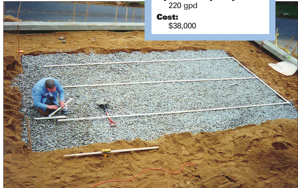
D.F. Clark employee Travis Good connects pipes for the pressure distribution field.
